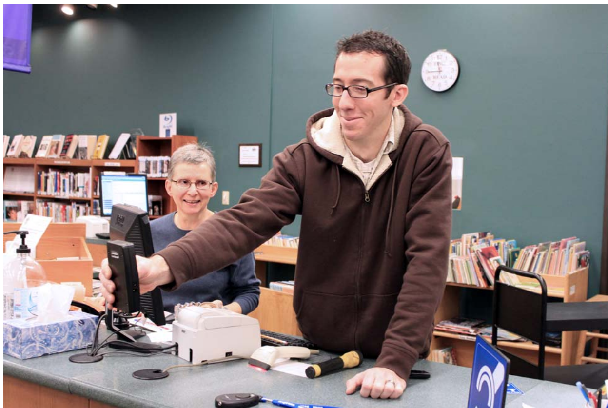
Photo caption: Circulation Department supervisor Marcia Stewart looks on as Ryan Enoch of Southern Tier Sight and Sound installs a Hearing Loop at the Southeast Steuben County Library.
